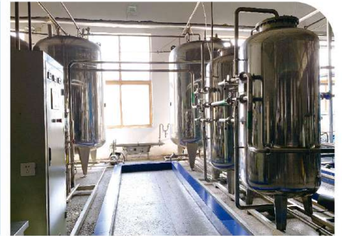
制水车间 ▶ Water making workshop
